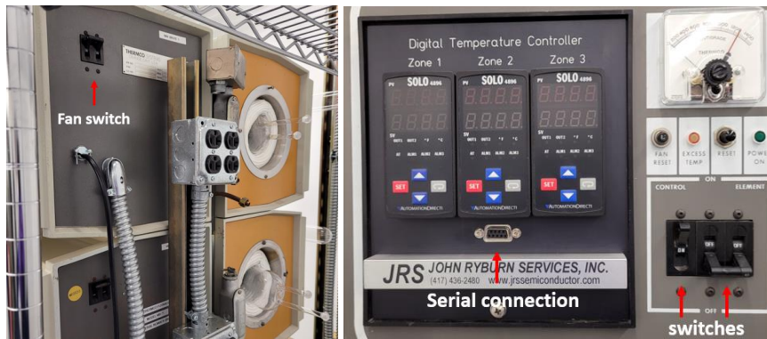
Figure 4: Fan switch (left), Power Switches & SOLO Controllers (right)
