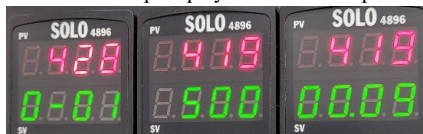
Figure 9: Control panel showing step number (left), set temperature (middle), and time remaining (right).
